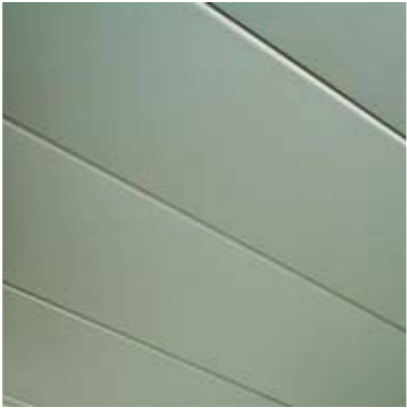
027 The false ceiling enhances the visual appeal of bathrooms and keeps service ducts concealed.
