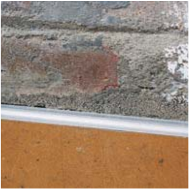
030 An aluminium U-channel is provided between the floor-skirting and the plastering of the wall for better finish. It also conceals cracks that may develop due to expansion.
