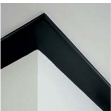
046 Wooden cornices that run along the ceiling conceal fire-fighting sprinklers even as they provide better finish to the rooms.
