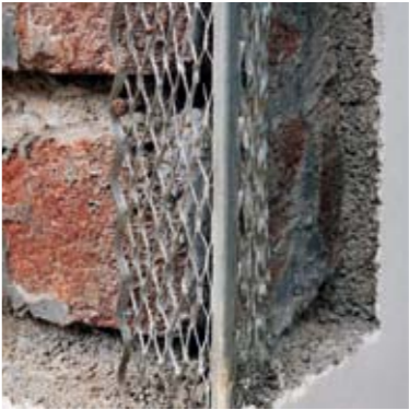
031 A GI mesh is embedded along corners of walls while plastering. This prevents chipping of edges and goes a long way in keeping the walls in great shape.
